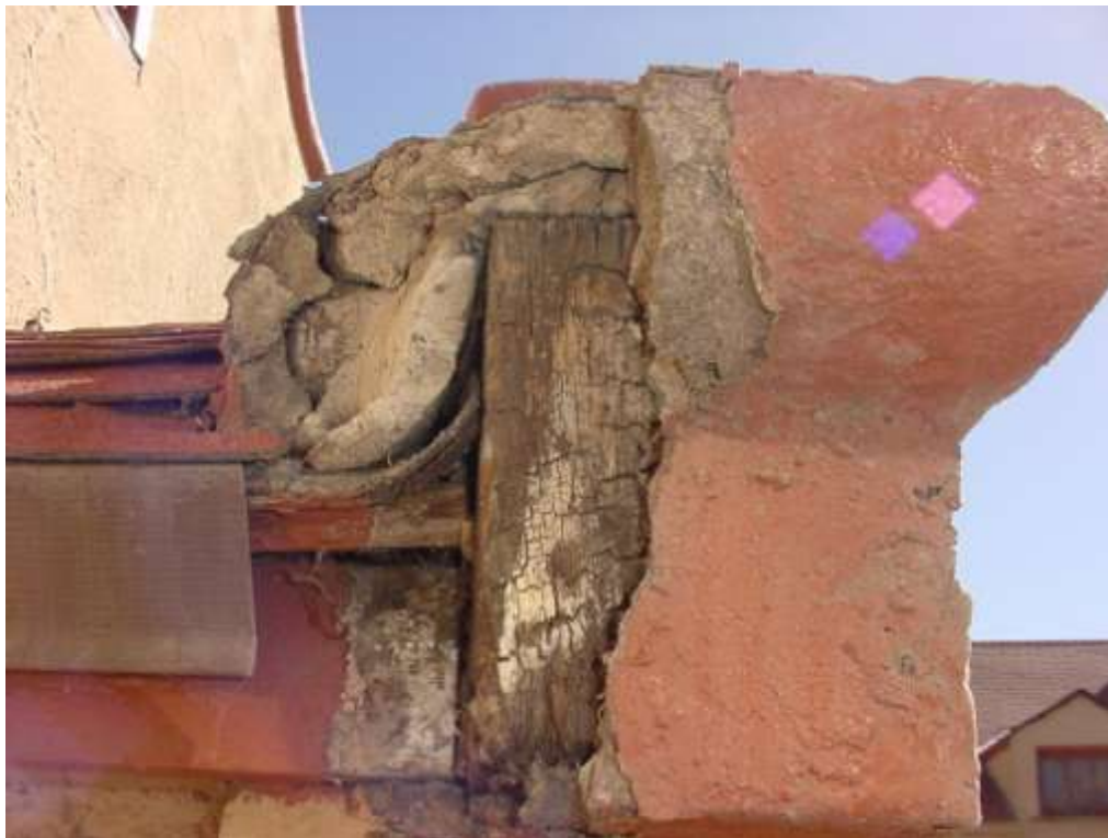
Wood rake boards and cement mortar trim at the west side of entry wall.
