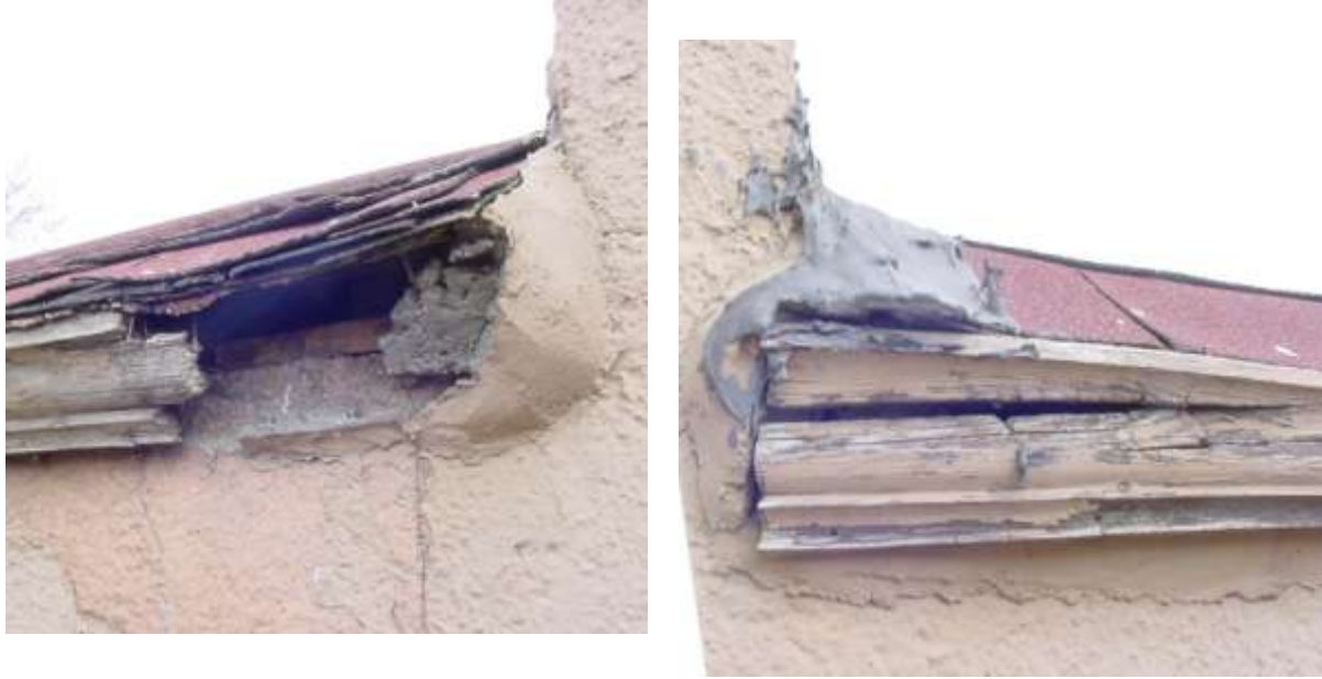
Deteriorated wood eave trim board in two locations at west wall of Parish Hall.
