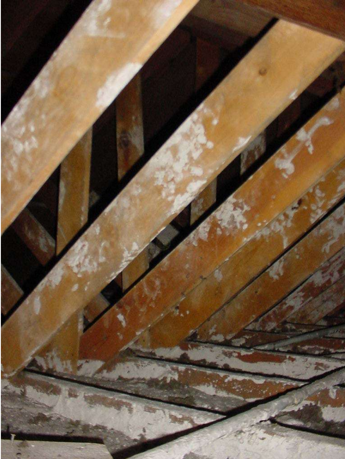
Roof trusses at Parish Hall. Note plaster-like powdery substance.
