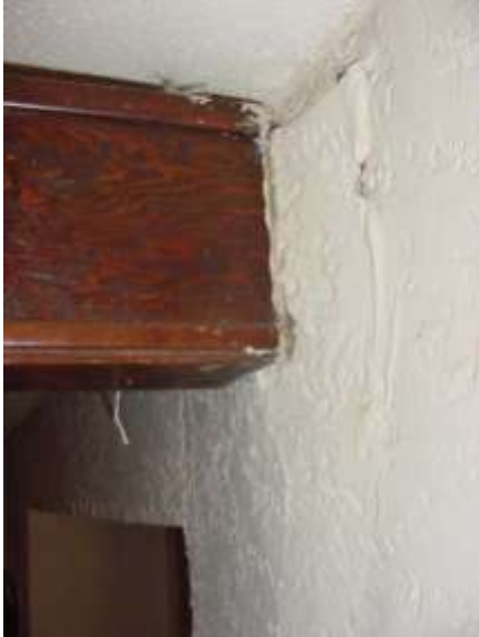
A close-up view of the Sanctuary decorative false beam. The beam does not bear on the Sanctuary side wall. Rather, it is merely toe-nailed to the structure. A look beneath the plaster revealed 2x blocking and celotex-type insulation board.
